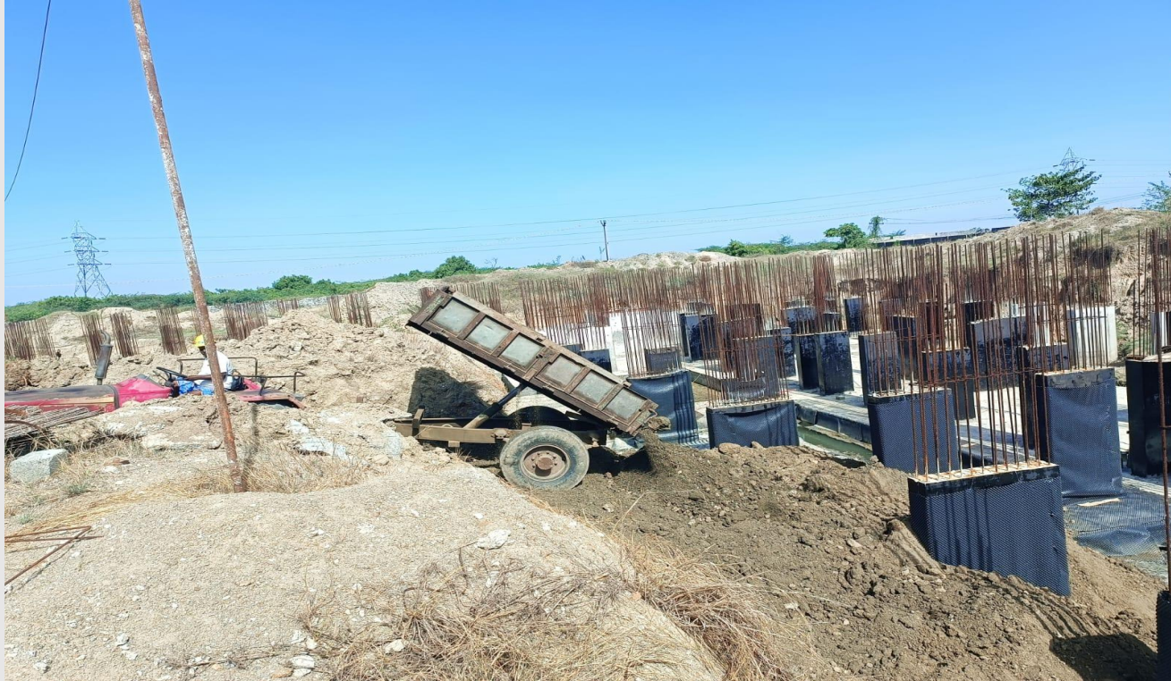
South side waterproofing completion area 1st layer soil filling works in progress
